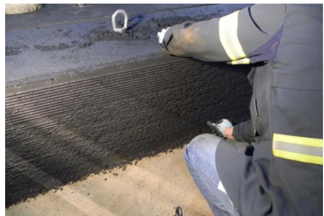
Figure 11. Compaction hardness and homogeneity.
